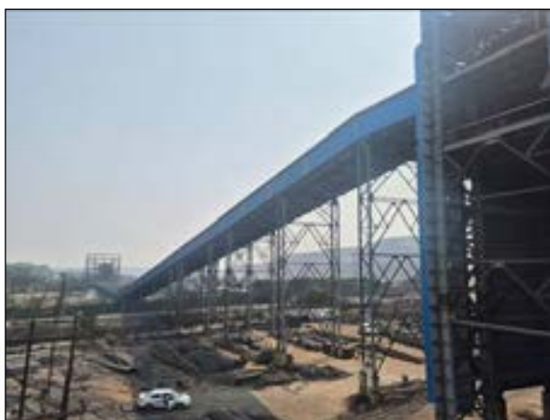
Figure 7: Conveyor system of CHP Construction (Design Scrutiny)
